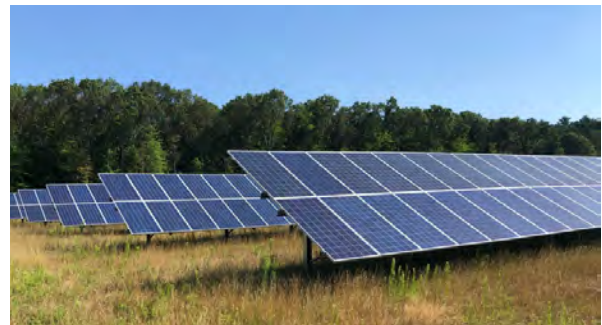
Eau Claire Energy Cooperative's 872 kW community solar array.
