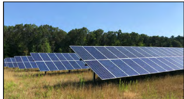
Eau Claire Energy Cooperative's 700 kW community solar array.
