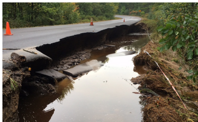
Figure 1. November 22, 2016. County Road G near Hathaway Creek.
