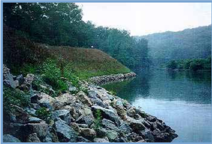
Figure 53: Riprap bank armoring for channel stabilization, Little Miami River, Ohio.
