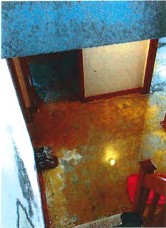
Figure 2 Photo of damaged basement
