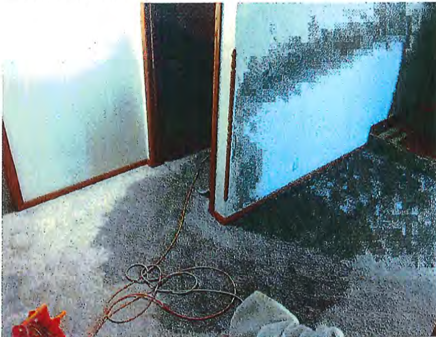
Figure 1 Photo of carpet and baseboard damage
